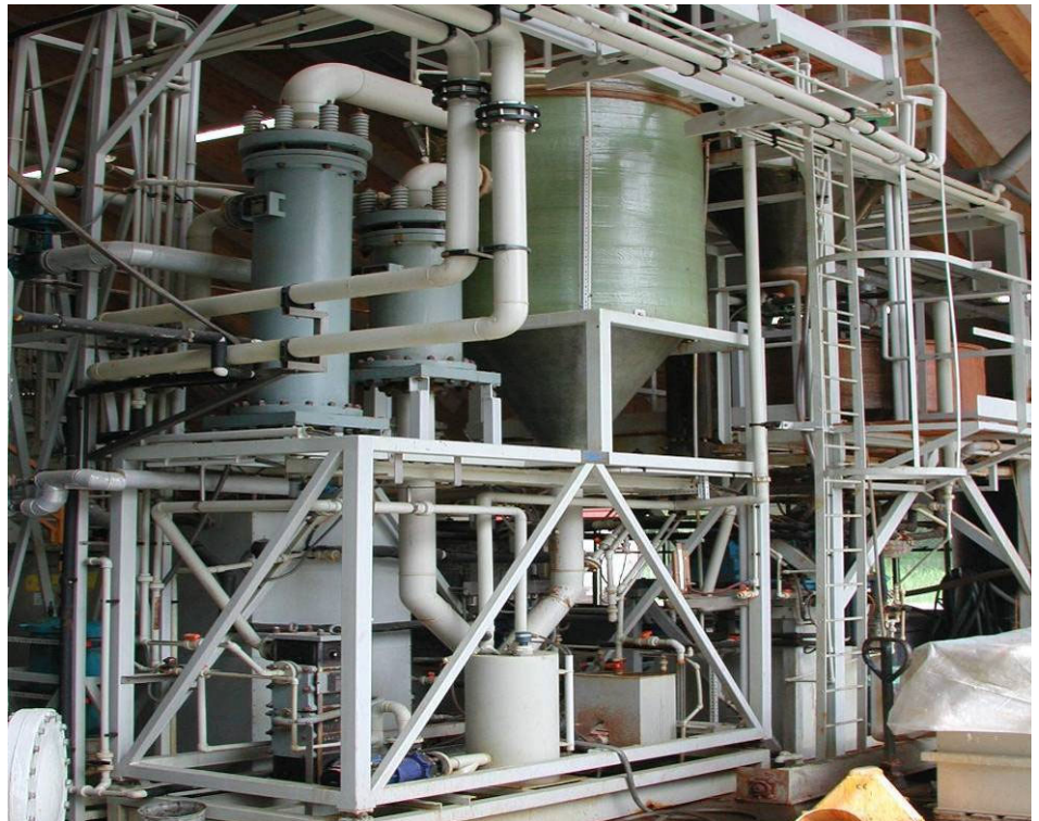
Fig. 1: view of the GALVASPLIT plant at Thommen-Furler AG in La Chaux-de-Fonds
